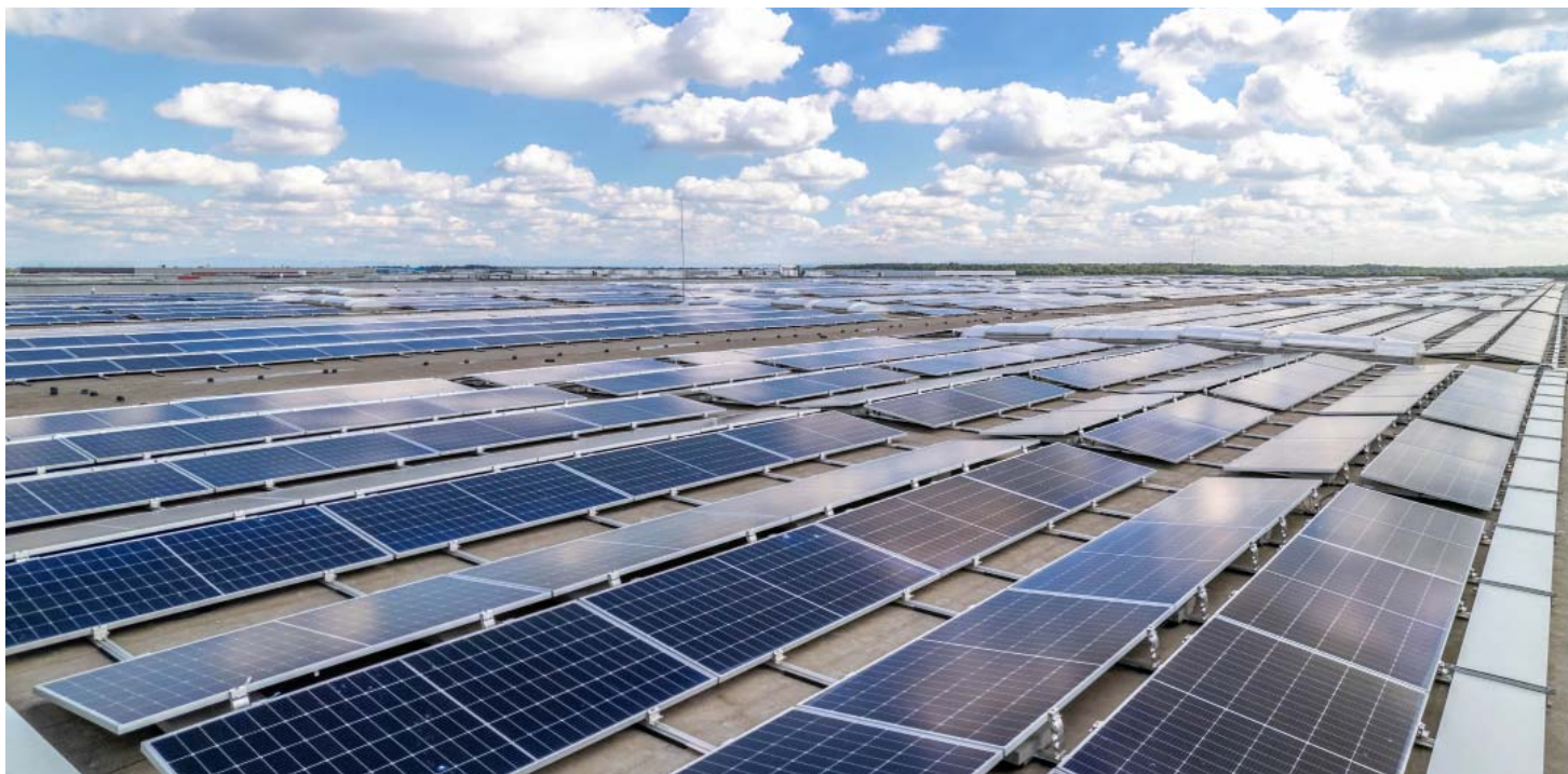
VGP Park Timisoara, solar panels
