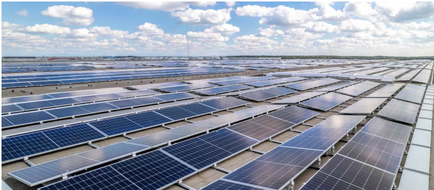
VGP Park Timisoara, solar panels
